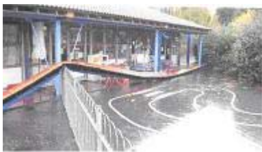
the fallen fascia
