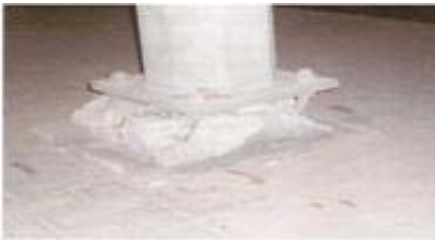
improperly installed and damaged base
